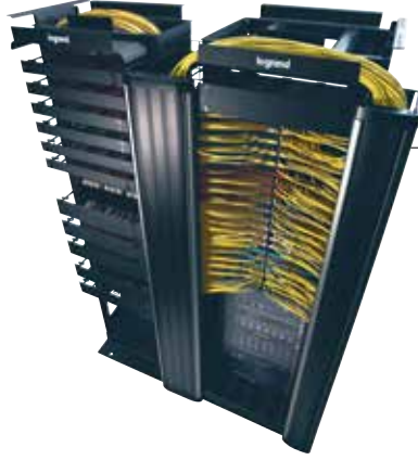
LCS 2 patch panel ve patch cordlar ile 0 464 06 + 0 464 27 + 0 464 26 + 0 464 18 + 0 465 70
